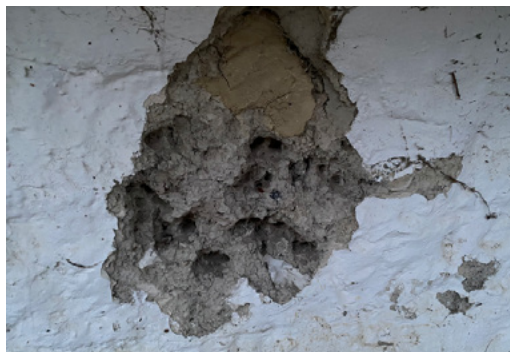
Fig 5. Section of cob wall in poor condition
