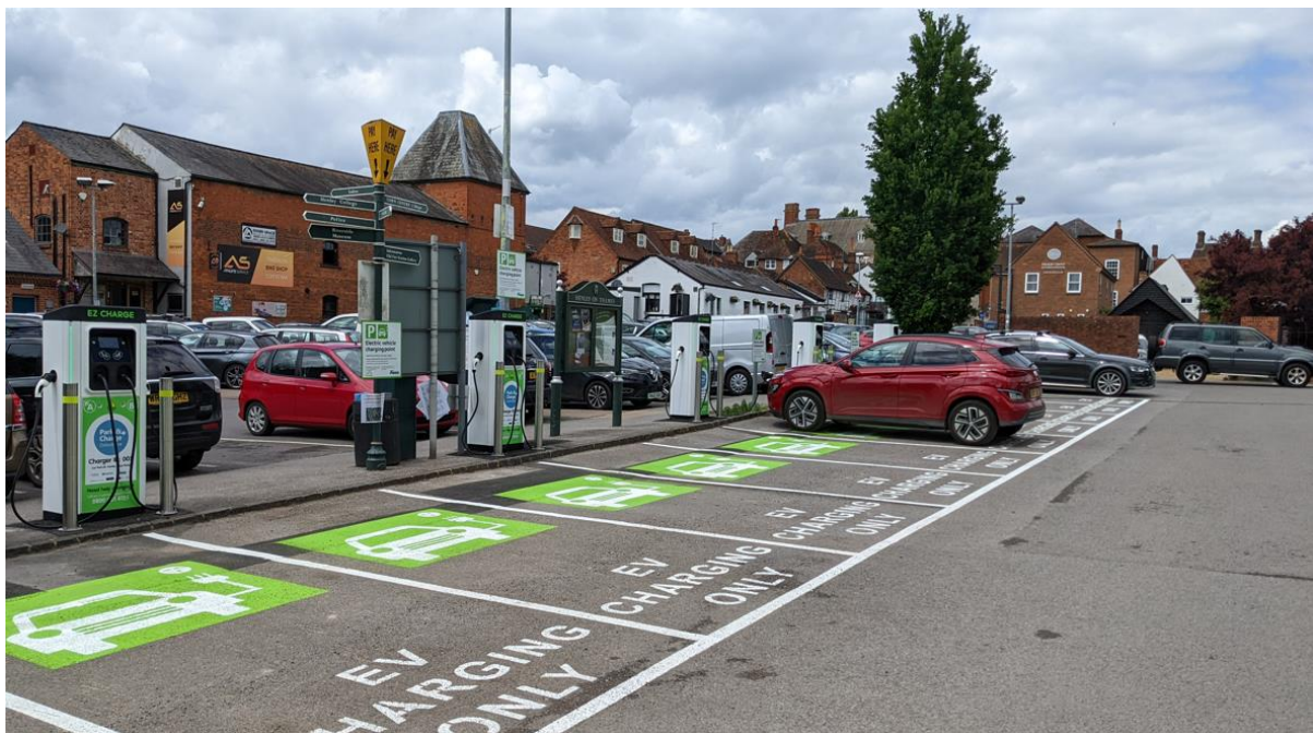
Figure 1 EV chargers installed in the Market Place car park in Henley
