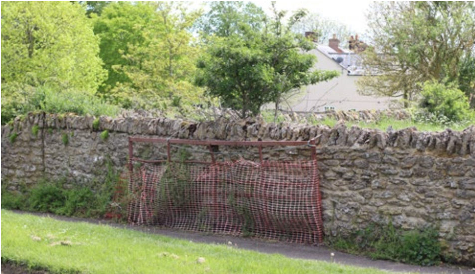
Fig 31. Damaged stone wall enclosure on Upper Green
