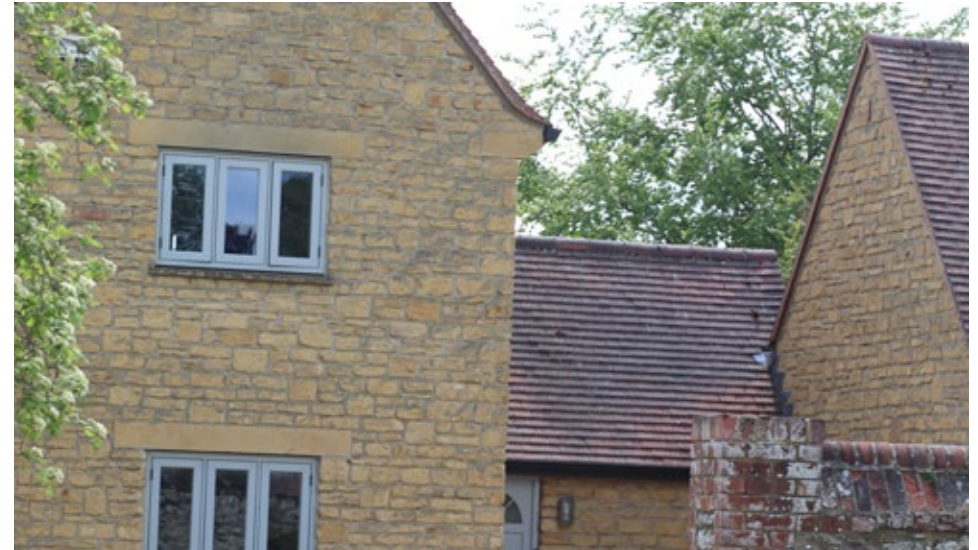
Fig 32. This modern house uses an inappropriate iron-rich Marlstone which has weathered to a mustard yellow colour
