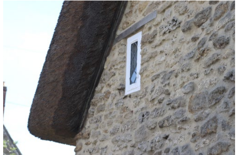
Fig 34. An example of good repointing using a lime based mortar, tamped back from the masonry face
