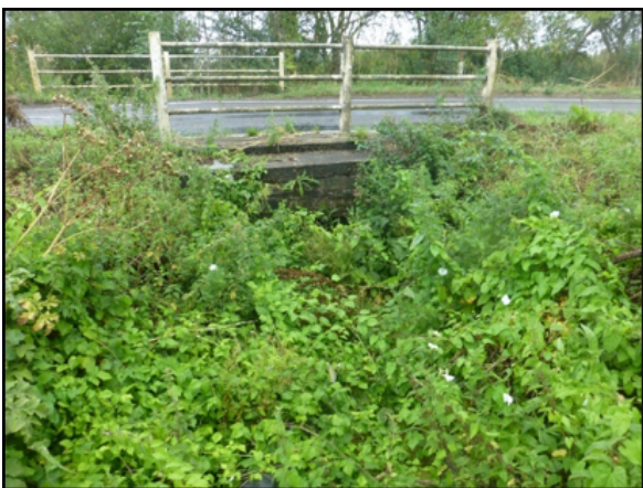
View from the end of 373/12 where the designated Right of Way meets the north end of 373/31 and Appleford Rd, B4016. A large diameter black pipe crosses the path and is a tripping hazard.
