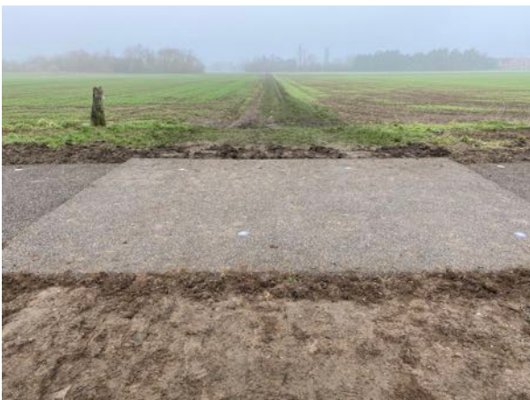
View west on the junction between the Cycle Track on Kelaart's Field and Milton's FP 299/4. Milton's FP 299/1 crosses just the other side of the post along the edge of the field in Milton Parish. 299/4 is part of the Vale Way and OCC Promoted Path.
