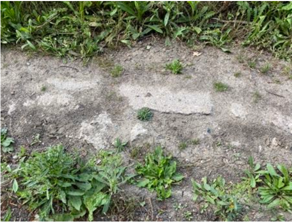
Broken slabs of concrete along BOAT 373/9, not reinstated after works by Thames Water.
