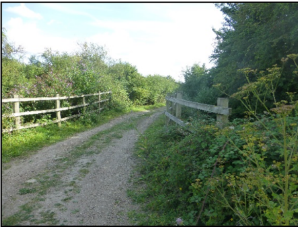
View of 373/10 south where it turns right, and crosses the culvert for the drainage ditch installed 2015 as part of the permitted landfill operations.
