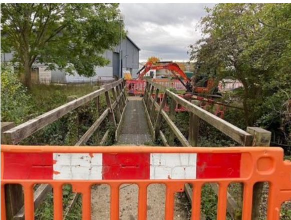
View south, of the old bridge over Moor Ditch, prior to its demolition 2020. This bridge is used in lieu of the older Moor Ditch bridge at the end of Milton's FP 299/1 and FP 299/2.
