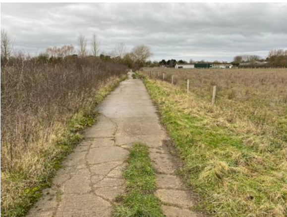
View west along 373/10, Old Wallingford Way toward the Recreation Ground on the left and Cross Trees Farm buildings on the right.
