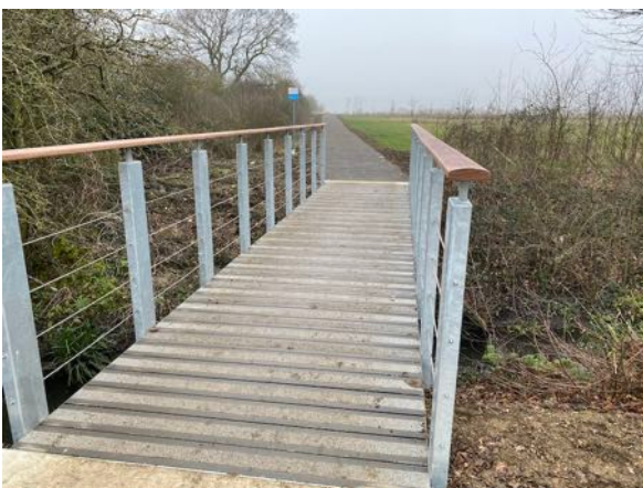
New bridge over Moor Ditch completed 2020/2021. The bridge connects MEPC's Milton Park with the shared use Cycle Track and Milton's FP 299/1 and FP 299/2.
