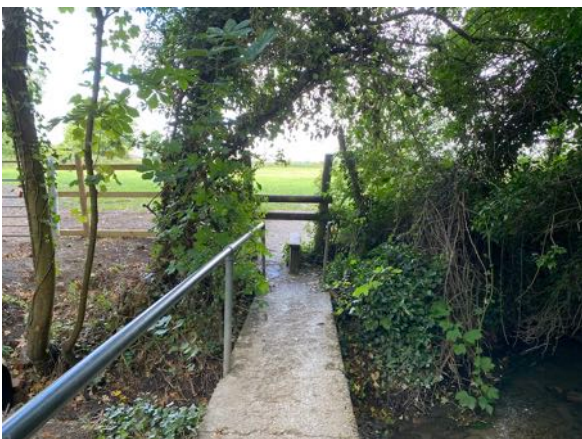
The concrete footbridge is over a ditch running into the Ginge Brook.
