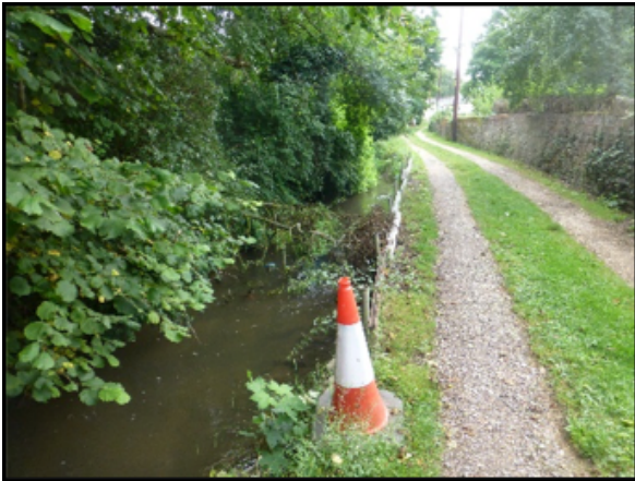
Ginge Brook showing damaged bank between House No. 2 and 4 Ginge Brook
