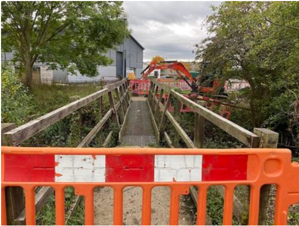
View south, of the old bridge over Moor Ditch, prior to its demolition 2020. This bridge is used in lieu of the older Moor Ditch bridge at the end of Milton's FP 299/1 and FP 299/2.
