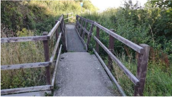
View north, of the old bridge over Moor Ditch, prior to its demolition 2020. This bridge was used in lieu of the older Moor Ditch bridge at the end of Milton's FP 299/1 and FP 299/2.
