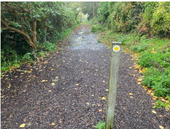
View from Old Wallingford Way, Byway 373/10, taken Dec 2020. The path was excavated to allow Magnox to remove a pipe in 2019. As a result of the work the path can now be muddy, made worse by the use of wood chips, which are already rotting adding to the problem.
