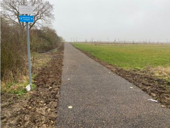
View back north along the new shared use Permissive Path Cycle Track over Moor Ditch from Milton Park, also used to connect to Milton's FP 299/1.
