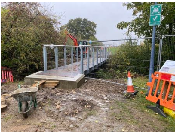
New bridge over Moor Ditch under construction 2020. The bridge is used for Milton's FP 299/1, FP 299/2 and the shared use Cycle Track, from the end of Milton Road in Sutton Courtenay and goes across the westside of Kelaart's Field, in the Parish of Sutton Courtenay.
