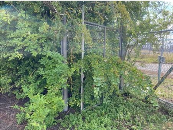
Closeup of fence/gate across the Bridleway. The remaining east/west section is inaccessible.
