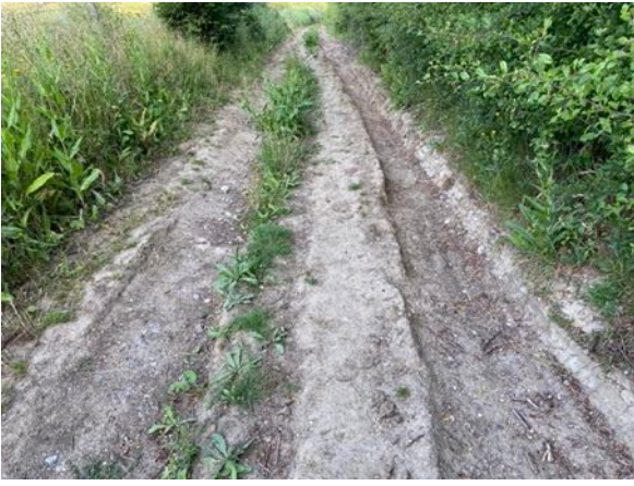
View back west, just after the dog-leg (double bend). Deeply rutted with slabs of broken concrete, remnants from the concrete roadway broken up by Thames Water in 2018.
