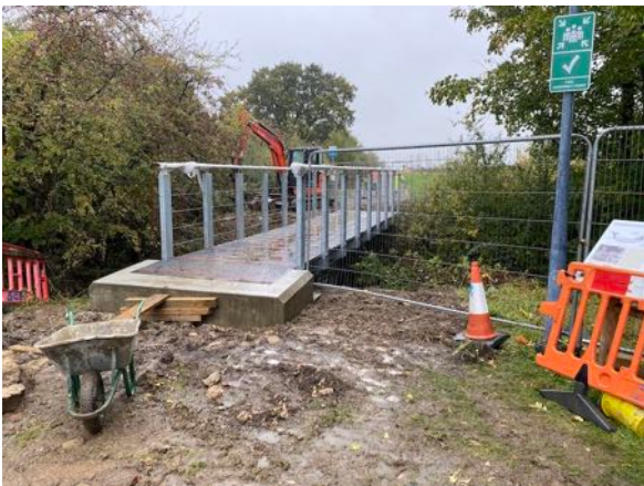
New bridge over Moor Ditch under construction 2020. The bridge is used for Milton's FP 299/1, FP 299/2 and the shared use Cycle Track, from the end of Milton Road in Sutton Courtenay and goes across the westside of Kelaart's Field, in the Parish of Sutton Courtenay.
