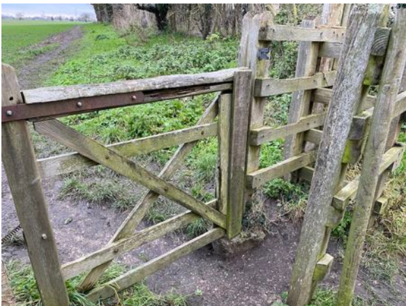
View west, along FP 373/16, across the Kissing Gate next to Ginge Cottage. The kissing gate is very small and in poor repair.
